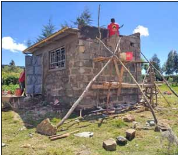
The new school kitchen at the Primary School Sision is now completed
